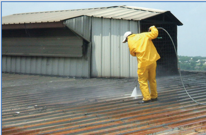
Prepare the roof. Prep and clean the roof, removing dirt and debris.
